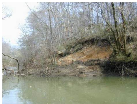
March 13, 2003. A large bank slump deposits tons of sediment into the Cahaba mainstem.
